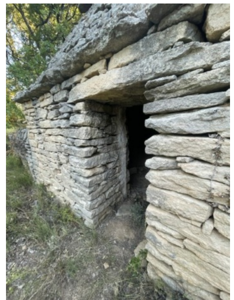
A close-up of the borrie (top of page) captures the fine dry stone construction in the doorway.
