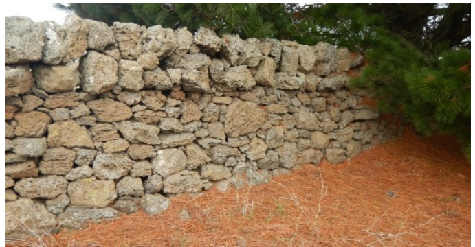
Galloway wall at the Corangamite Dry Stone Wall Site near Derinallum. Single stone above coverband.
