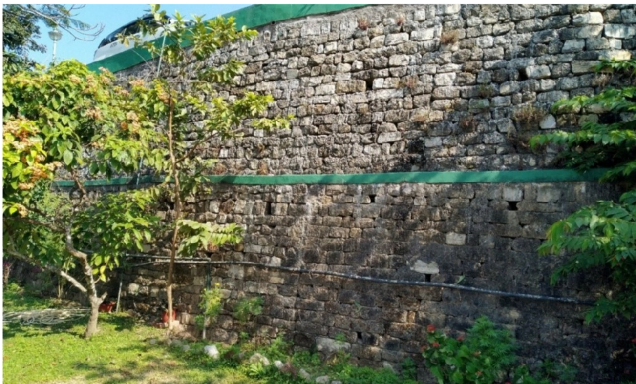
DSW below the terrace of the main drive and front entrance, possibly the oldest location at Glenburn but with probably not much nineteenth century walling surviving and mortared joints at the very top.
