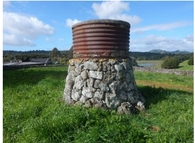
Dry stone tank stand (Kamo). The evident concrete is lining the rusted tank!
