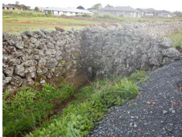
Original wall in the estate showing drain, smooth and un-restored wall end where the gap was made for the road.
