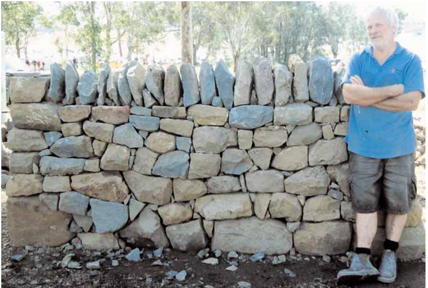
The finished wall proudly displayed by Kim Barnfield, stone mason and DSWAA member; NSW
