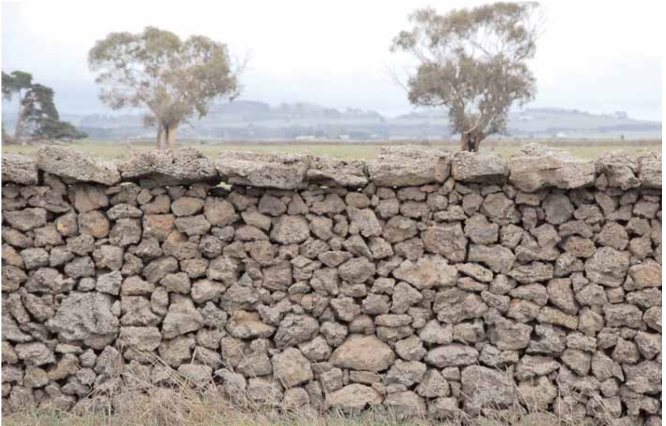
A typical dry stone wall in the landscape of Victoria's Western District
