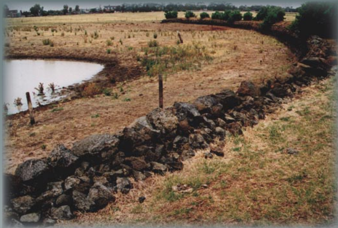
Large dam with extensive stone retaining wall attributed to W.J.T. Clarke one of the early pastoralists in the State of Victoria. By early 1837 the Werribee plains were fully stocked with sheep to a distance of forty kilometres inland from the coast of Port Phillip Bay. Photography – Jim Holdsworth
