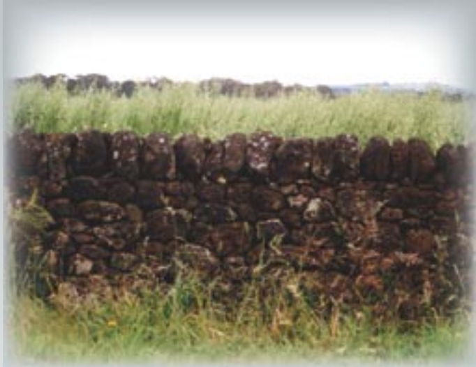
Timeless walls. New walls. Unfinished walls. To the passer by near Wallace this wall appears to be an old, but finely crafted wall, in poor condition. However, the pile of rocks nearby, represent the events that surrounded its construction by Nathan Perkins in the early 1990s as a demonstration event at a Draft Horse Festival.
