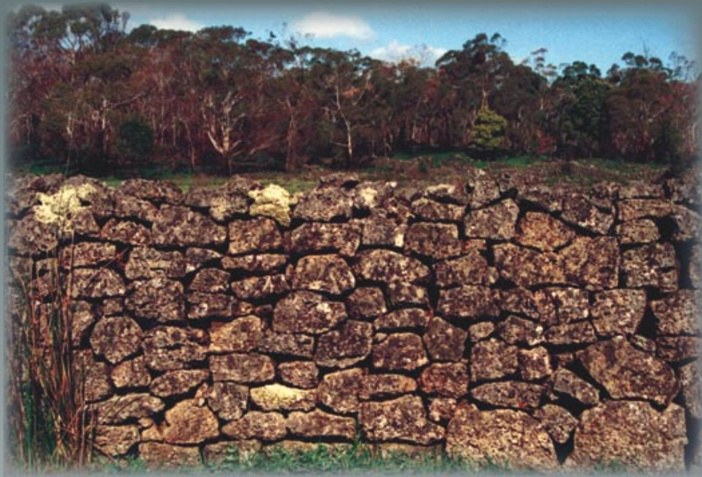
A fine example of dry stone wall construction, located in the Parishes of Condah & Dunmore, north-east of Heywood, Victoria.
