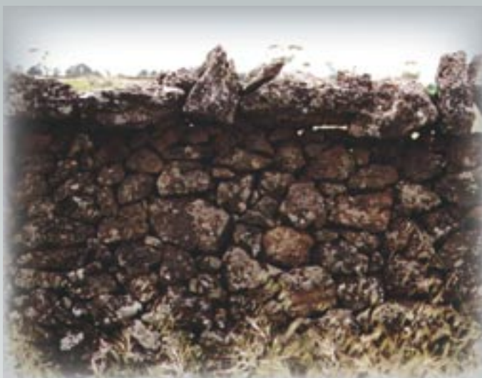
Cock and Hen – Wallers often varied the copestone configuration to provide some uniqueness in the wall. This is an example of a Cock and Hen from Rands Road, Pomorobeit North.
