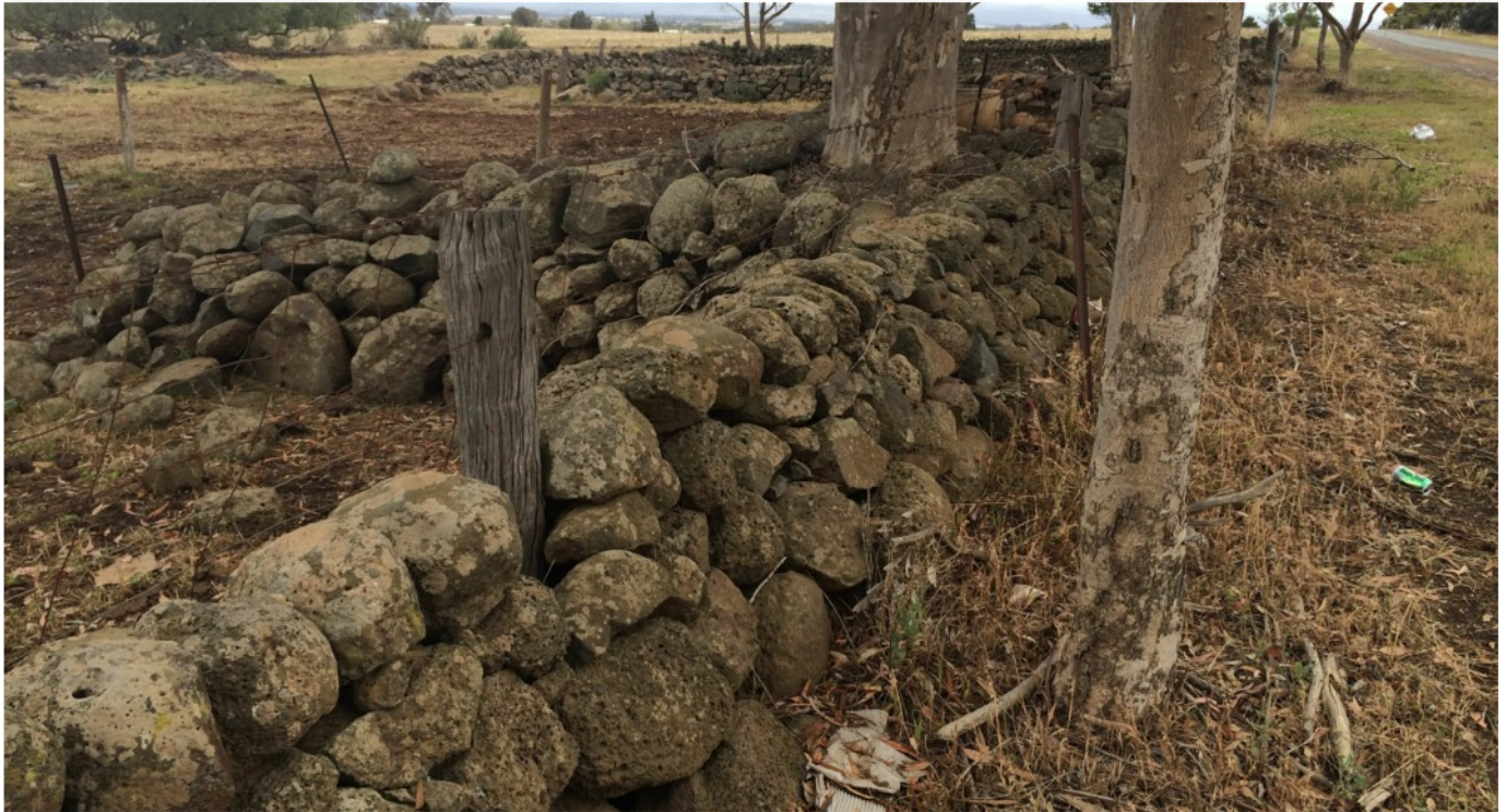
Mt Cottrell Road, owned by Melton Council, has dry stone features such as walls, a stockyard, a dam and a stone-lined well all in a confined area
