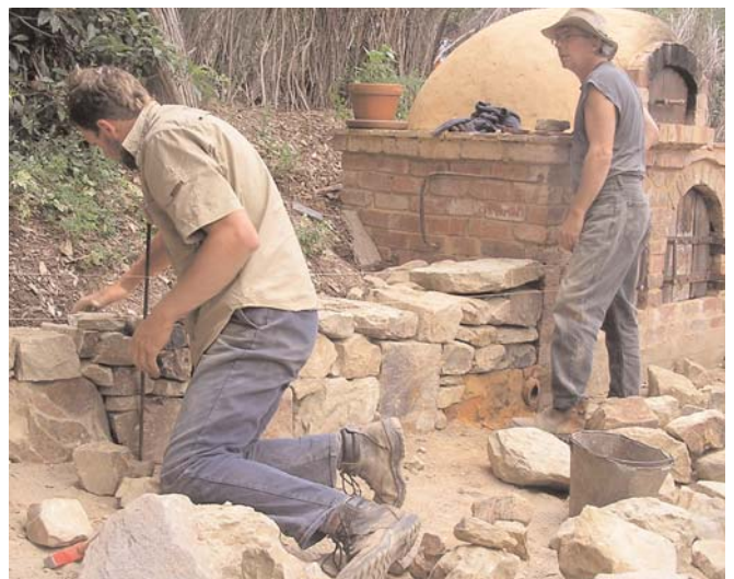
Al and Gerhard hard at work on the dry stone wall made of local sandstone.
