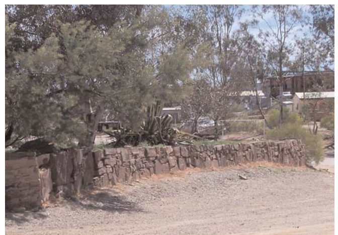
A recent dry stone wall – note slabbed stones, a unique feature of Andamooka walling.
