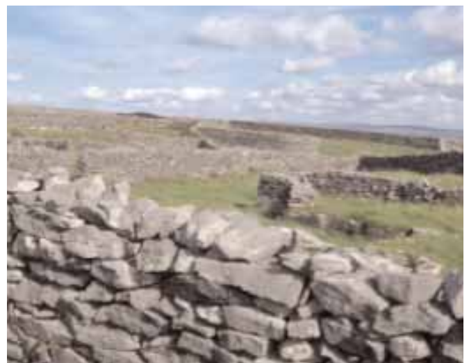
1. Building dry-stone retaining wall. 2. Four-metre-high dry-stone retaining wall 3. Walled fields on Inis Oirr
