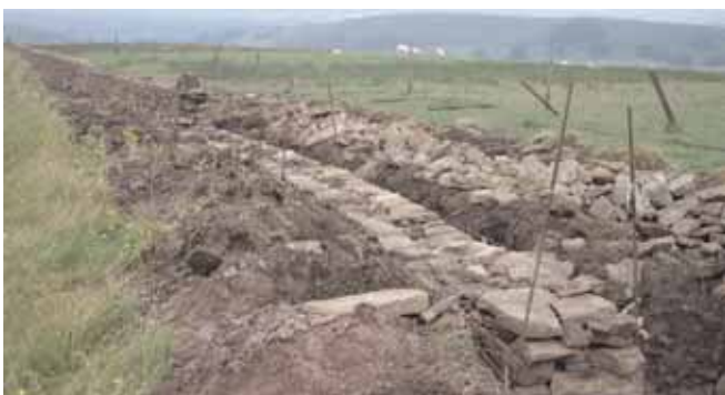
Wall in the process of being repaired in the Derbyshire Peak District, UK 2012
