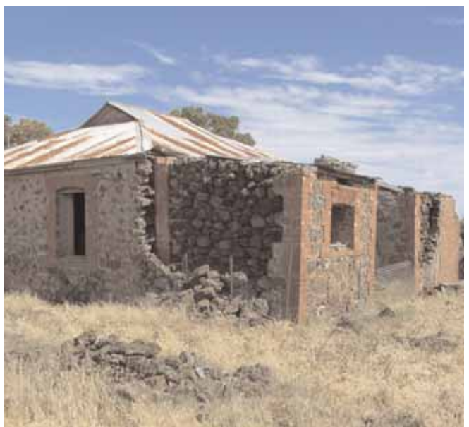
Ruin of First World War soldier settlement cottage at the Thompson property showing how the internal walls were made from the surrounding field stone
