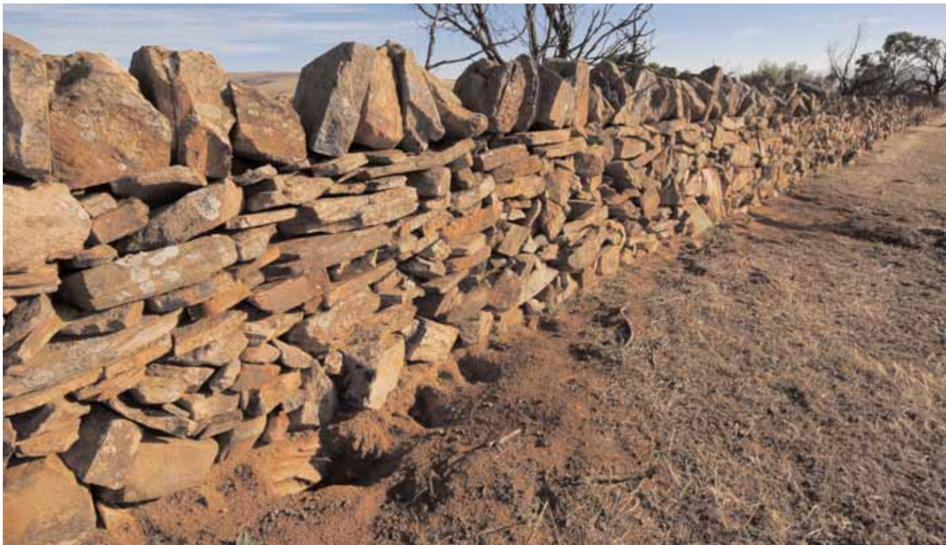
Eden Valley, South Australia, showing damage done by rabbits undermining wall
