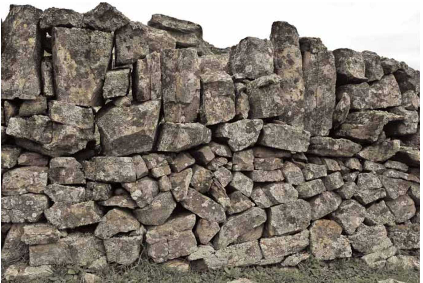
Camel's Hump wall, Farrell Flat, showing Galloway style designed to thwart rabbits
