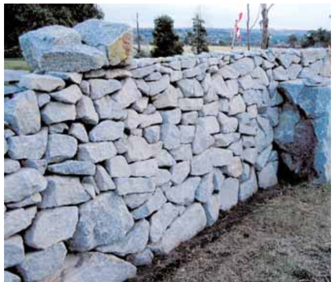
The wall is nearly complete – two large copestones can be seen on the top. When copestones have been placed along the entire top of the wall then the wall is complete Photo courtesy of Nick Platt
